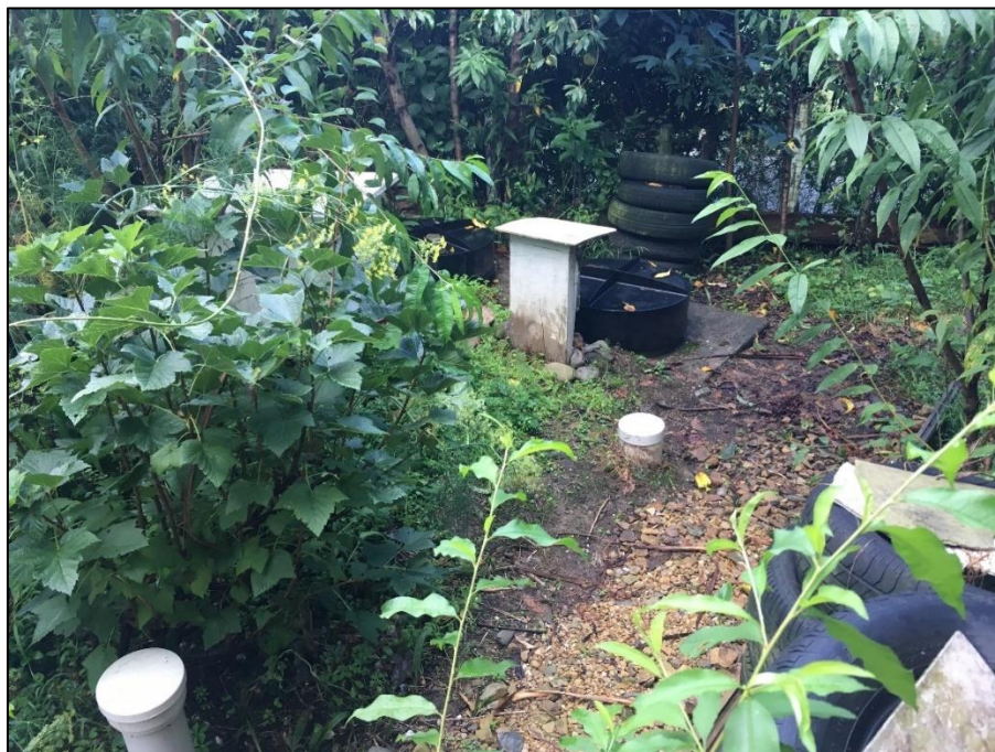
Primary settling tank and EcoWaste AWTS
