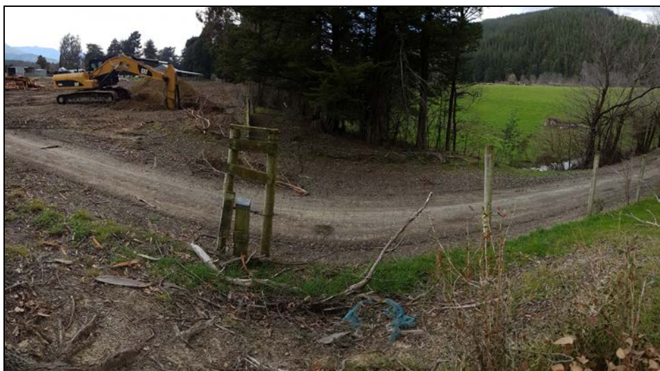
Photo looking west showing Test Pit E being excavated close to the Wairau Fault terrace bank (note fault follows the grassed hollow to the right of the photo)
