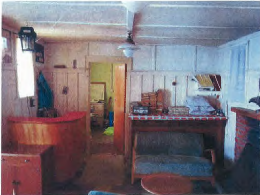
Internal layout - note subsidence in dividing wall
