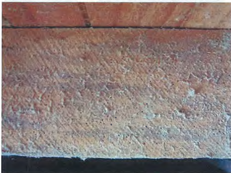
Borer in floor joist
